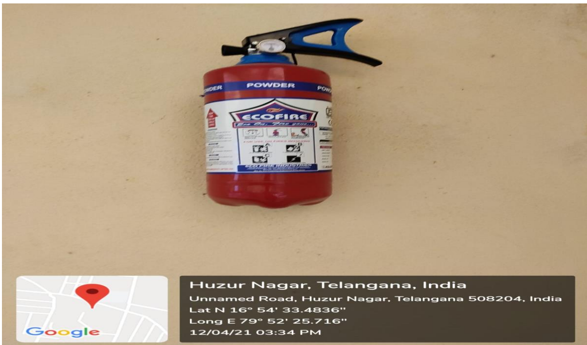
Fire Extinguisher at Auditorium of the GDC, Huzurnagar
